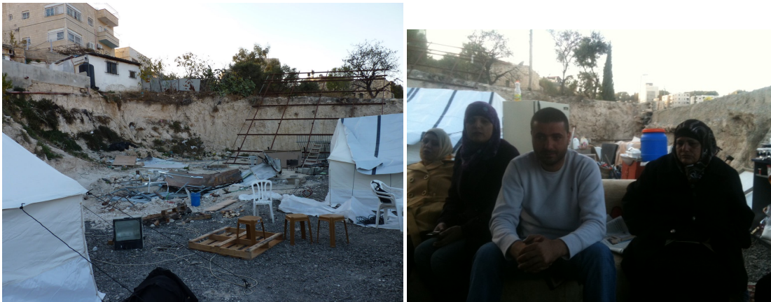
(left) Site of the demolished house of the Subuh family in Ras Al-Amud, East Jerusalem. (right) Subuh family members sit at the site where their house was demolished two days earlier, on 21 December 2010. ©ASF delegation
